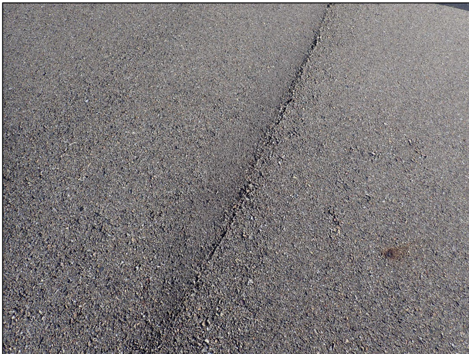
TW-10-02: L&T Cracking
